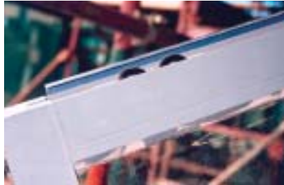
Retro-fitted angle section to prevent the sliding window from leaving its track.
