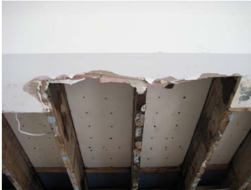
Water damaged flooring above ceiling
